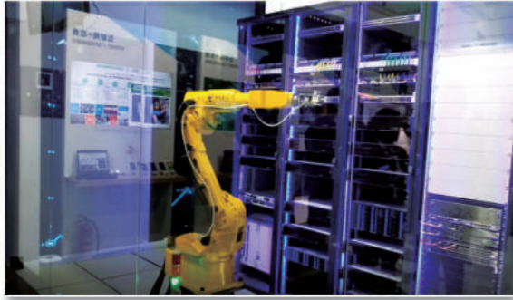
Emergency Handling in the 3C Industry Intelligent Data Center
