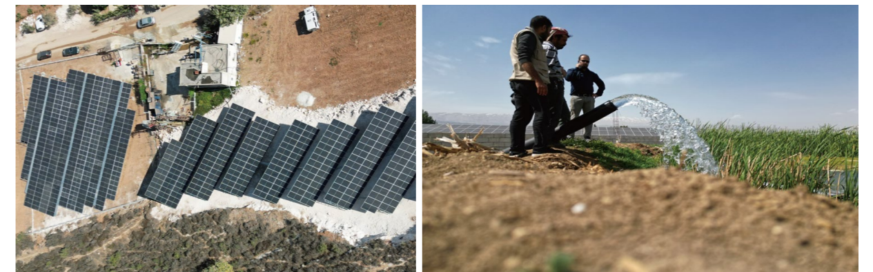
160KW Solar Irrigation Project in Lebanon
