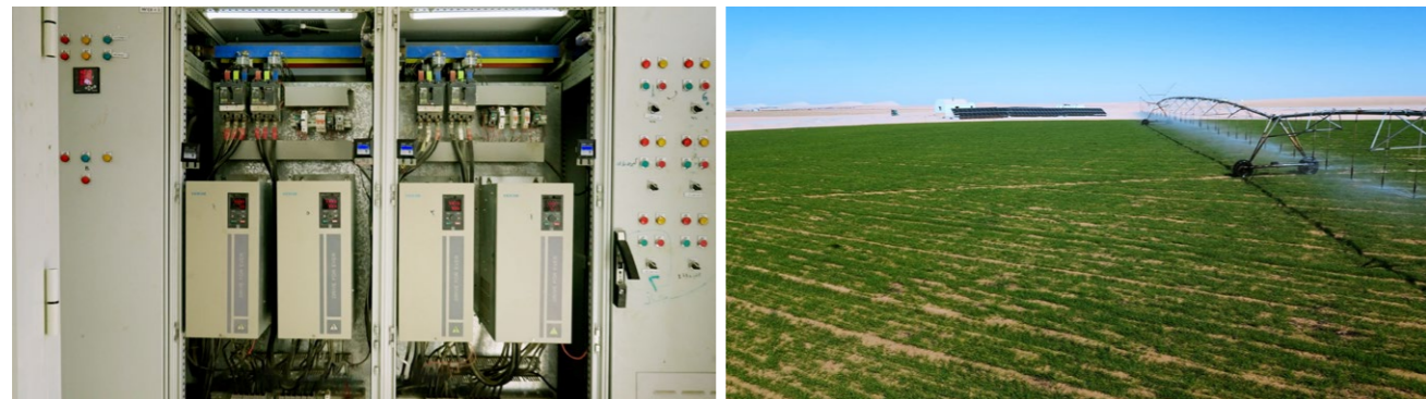
206 kW Solar Irrigation System in Egypt
